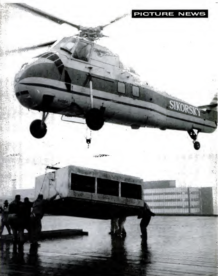
Copter handles big moving job. A helicopter spots a 3,400-pound heating unit here on the roof of Convair's new Atlas missile factory in San Diego. Making 70 quarter-mile trips, it brought 100 tons of heating and ventilating equipment in six hours. Conventional methods would have taken four weeks, required reinforcing the building for rigging.
